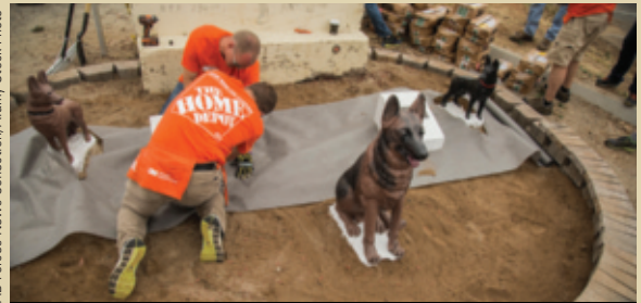
Volunteers with The Home Depot's Building Materials Department help to restore the memorial of Sergeant Adam Cann during the K9 upgrade project at Camp Pendleton.
