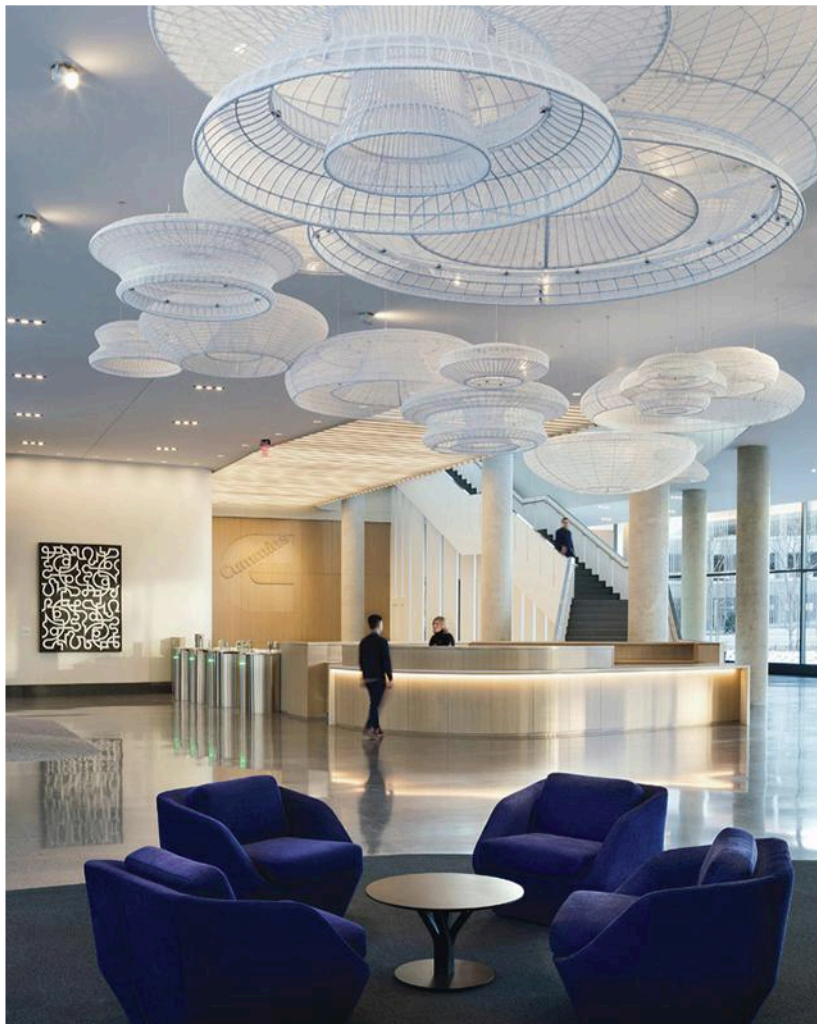
The light fixtures from GE Current introduce efficient LED lighting and IIoT sensor and data collection capabilities.
