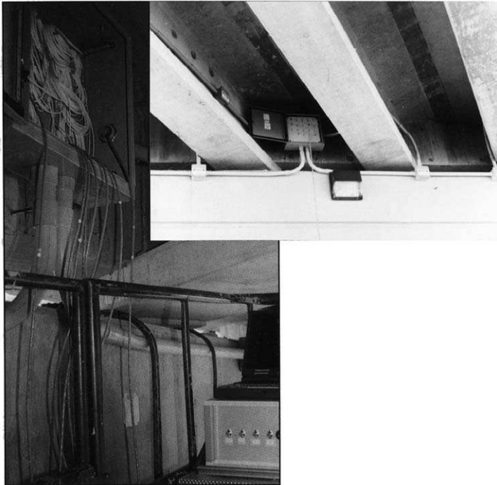
FIGURE 9.41. Two views of the junction box for the fiber optic sensor array of the Beddington Trail Bridge. Used with permission, ElectroPhotonics Solutions Corporation.
