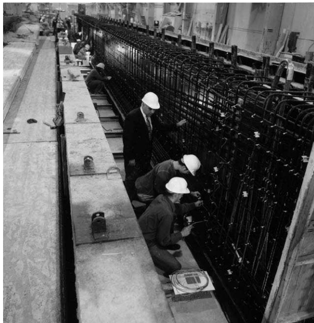
FIGURE 9.49. Installation of FBG sensors into the CFRP shear reinforcement frame for one of the precast concrete girders for the Taylor Bridge. Used with permission, ISIS Canada.
