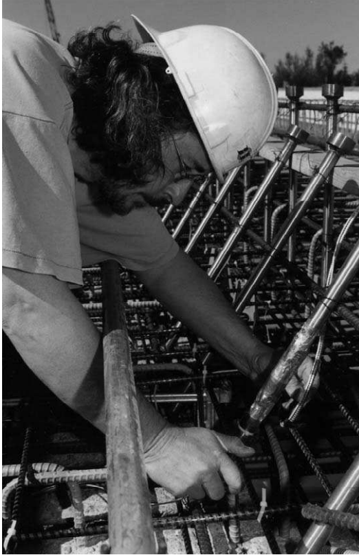
FIGURE 9.50. Installation of FBG sensors into the Taylor Bridge barrier-wall reinforcement frames. Used with permission, ISIS Canada.
