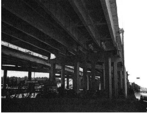
FIGURE 11.57. Photograph of I-10 Bridge over Las Cruces. From Idriss, R. L., White, K. R., Pater, J. W., Vohra, S. T., Chang, C. C., Danver, B. A., Davis, M. A., (1998), "Monitoring and Evaluation of an Interstate Highway Bridge Using a Network of Optical Fiber Sensors", Fiber Optic Sensors for Construction Materials and Bridges , F. Ansari (Ed). pp.159–167, © 1998, Technomic Publishing Co. Inc.
