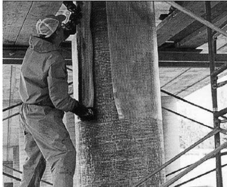
FIGURE 2.19. Repair and strengthening of a corroded concrete column by FRP material wrap. Used with permission, ISIS Canada.
