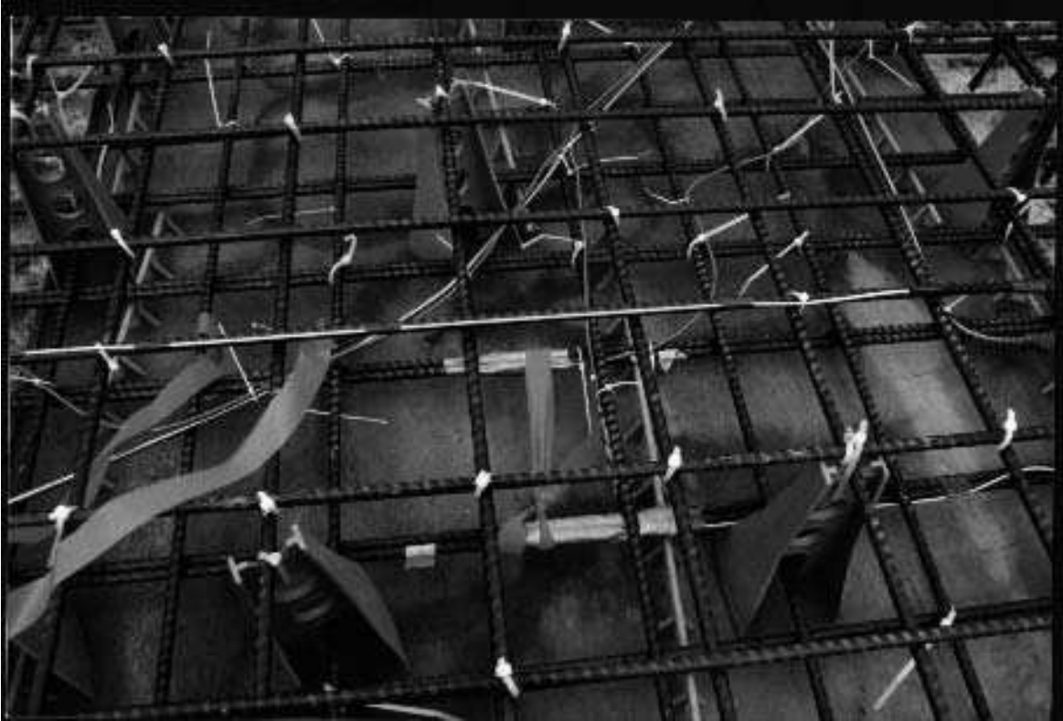
FIGURE 8.8. Several fiber optic instrumented rebars are seen within the mesh of steel reinforcement for a concrete structure. The optical fiber cables are routed along this mesh to the planned egress points for the concrete structure.
