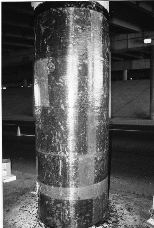
FIGURE 10.48. Installation of localized, long gauge-length fiber optic sensors into the FRP rehabilitation and strengthening wrap of concrete columns supporting the 401 highway in Toronto.
