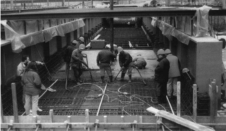
FIGURE 10.30. Installation of the fiber optic deformation measurement tubes during construction of the concrete deck for the new Moesa railway bridge, Switzerland. From Inaudi, D., Casanova, N., Kronenberg, P. and Vurpillot, S., (1997a), "Railway Bridge Monitoring During Construction and Sliding. SPIE, Smart Structures and Materials , 3043, San Diego, USA, 58–64.
