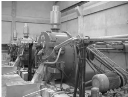
(g) Dewatering centrifugal
