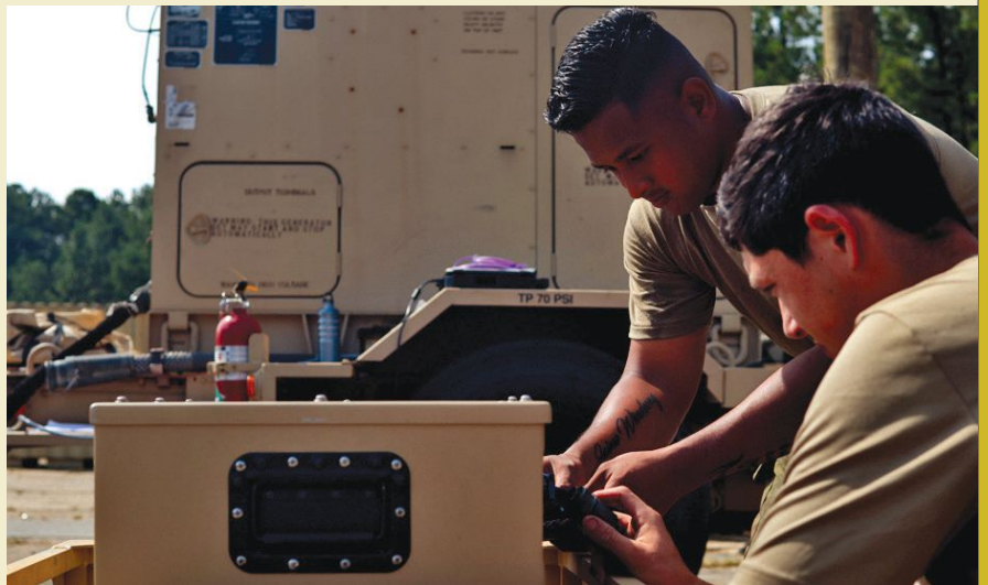
Soldiers test the hybrid power system microgrid at Fort Bragg, North Carolina.
